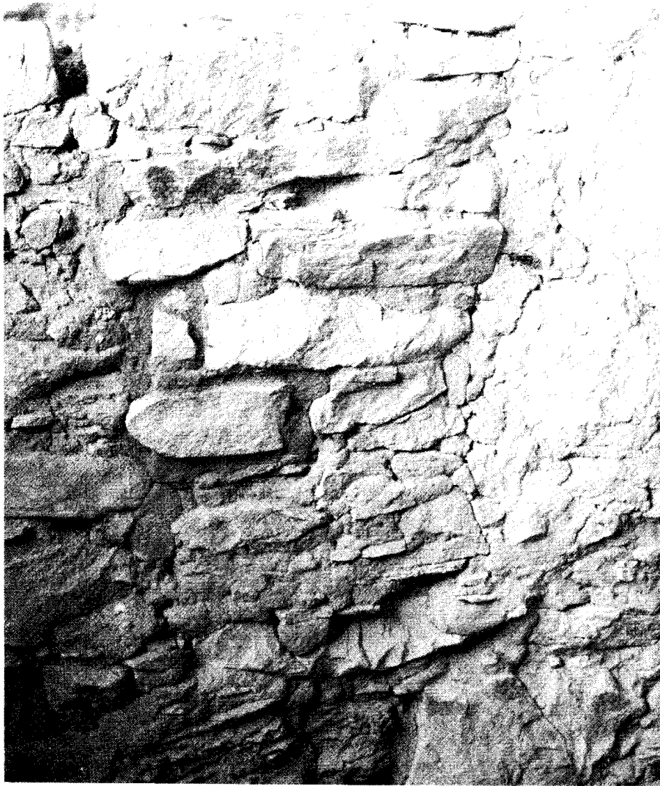
Figure 34 Plugged Entry in West Wall of Room 10
