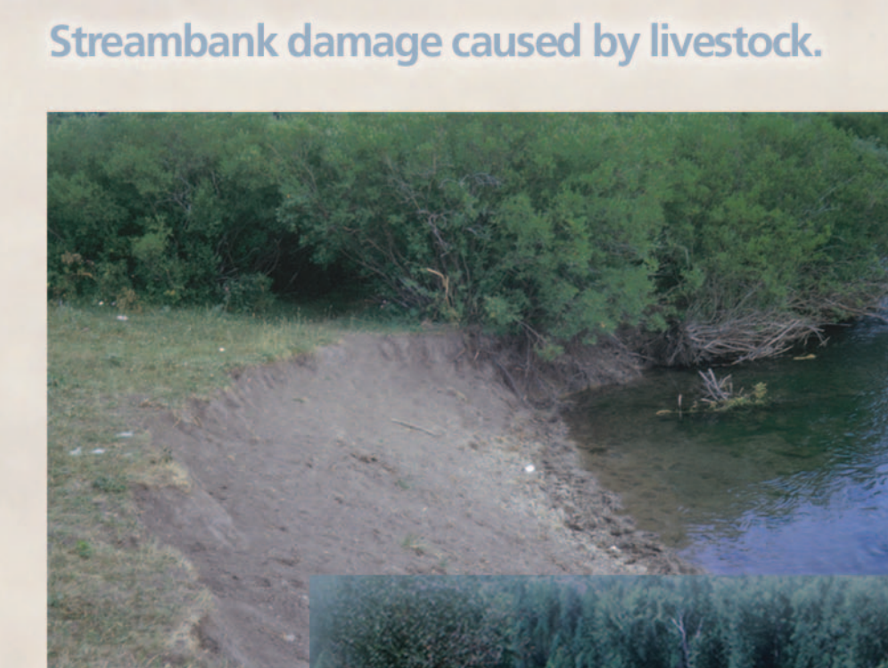
Streambank damage caused by livestock.
